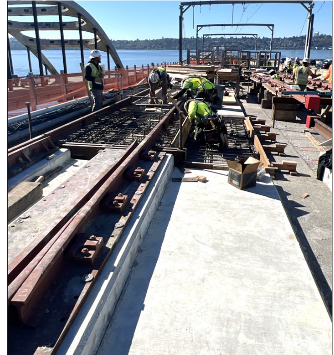
In progress plinth construction on the east approach to the Homer M. Hadley Floating Bridge
